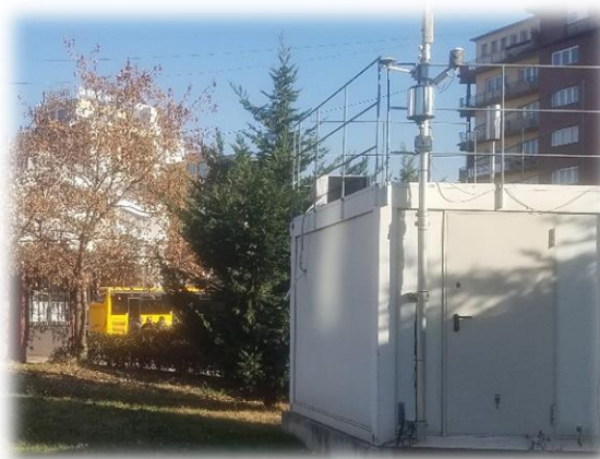
Fig. 4. Air Quality Monitoring Station in Prishtina (Rilindja)
